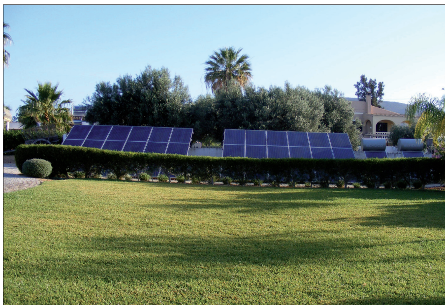
Fig. 2: Ground-mounted solar PV UPP in the Algarve region (Photo: L. Silva)
