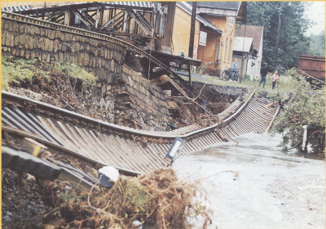
Destroyed railway near the station of Loučná nad Desnou under mined with water during the culminating flood. (Sunday, 20 July 1997)
