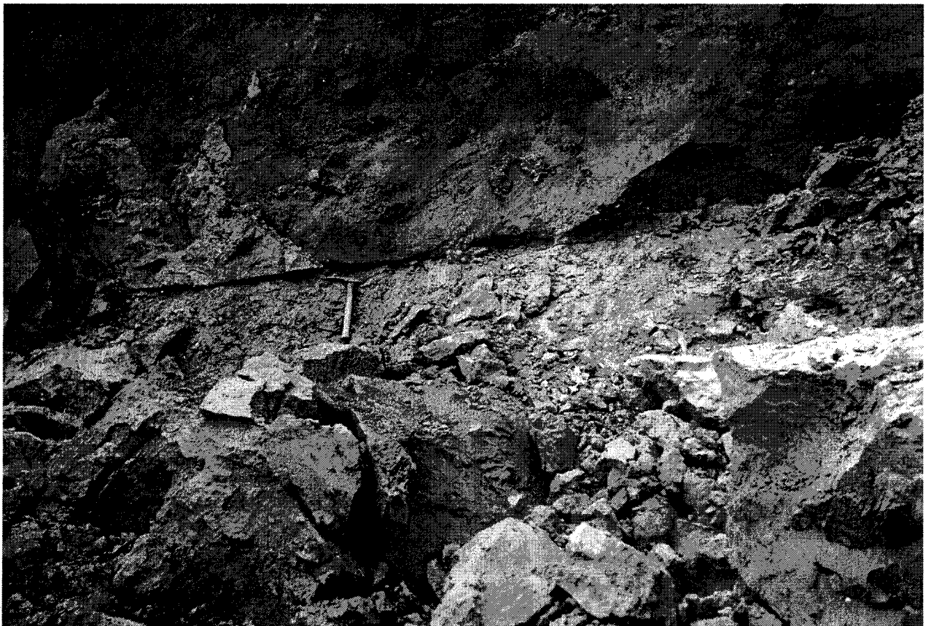
Fig. 16 The lithological boundary between calcareous clay and rock cover loess, pointed out by the dislocation along the slip area. The movement of a loess series part took down also the blocks of calcareous clay (to the left from the hammer). Photograph J. Karásek, November 1995
