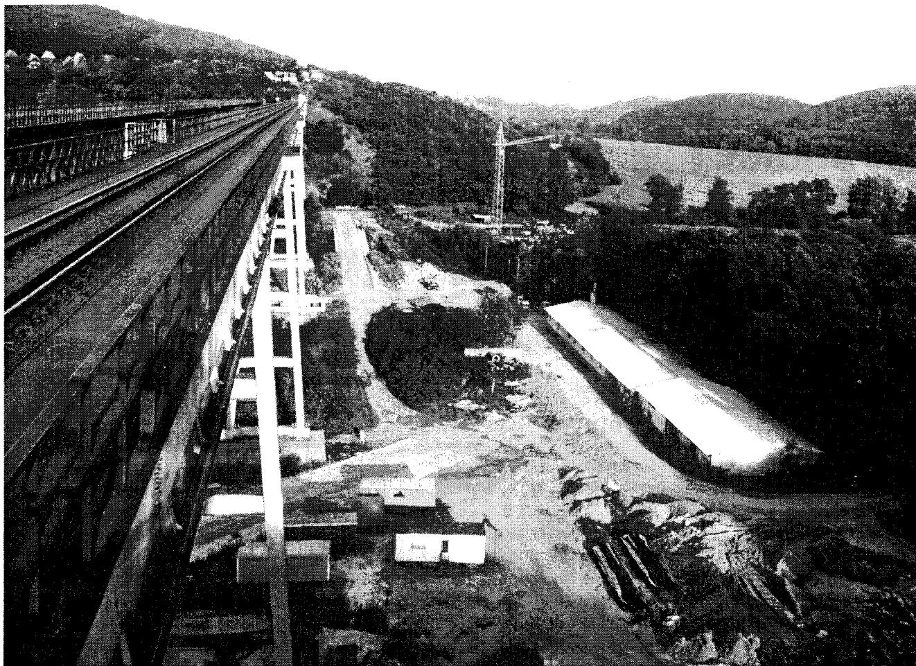
Fig. 2 The Ivančice viaduct across the Jihlava River valley. The western support is founded on piles in Miocene water-bearing sands, the northern support is fixed on the opposite side of the valley in crystalline massif. The tectonic Bránická kotlina (basin) with a broad floodplain and subsided Miocene sediments to be seen to the right of the bridge, to the left the structure of the old Ivančice viaduct. In the left background in front of the forest and summer houses there is a rocky slope bench bounded by a fault at the foot of the higher slope. Here the Jihlava River left a high river terrace. Photo M. Hrádek.
