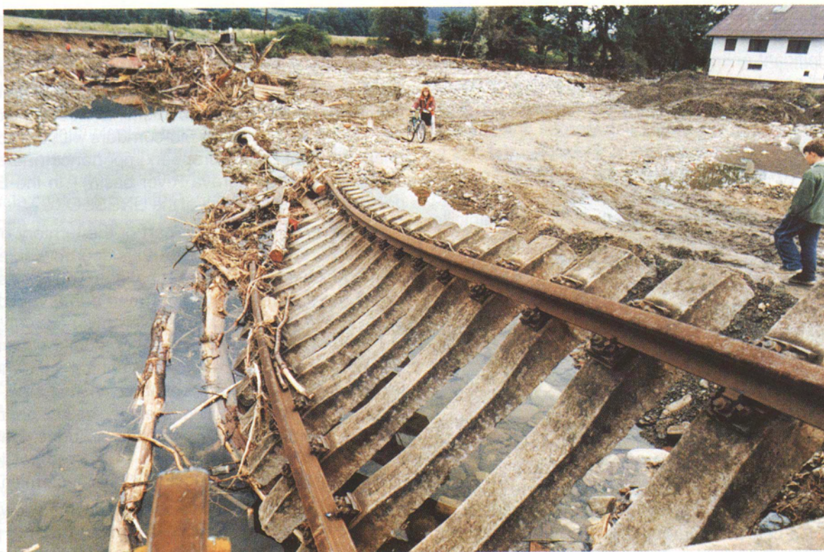
Fig.3: Ripped off rails in Rapotín, Šumperk district, 20 July 1997. Photo: V. Galgonek
