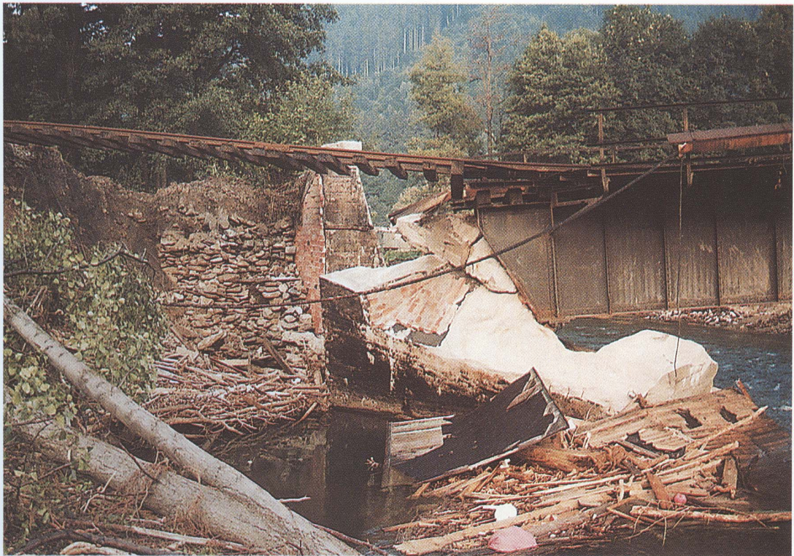
Railway bridge in Hanušovice after flood in July 1997
