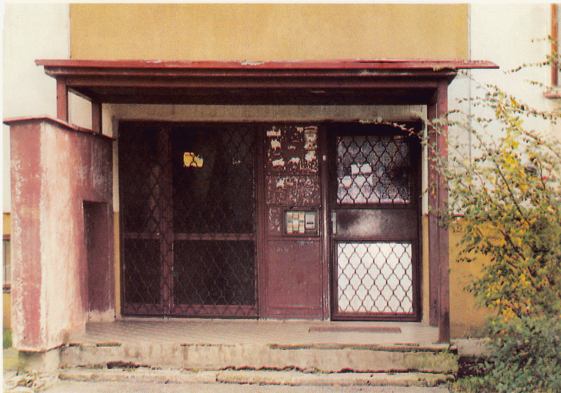
Untidy front door of a panel apartment house (Frýdek-Místek, housing estate Slezská)
