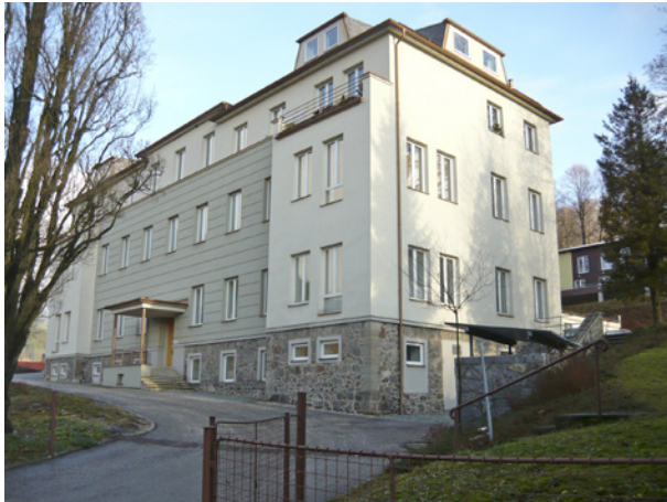
Fig. 3: Reconstruction of the former hospital into a recreational apartment house in Horní Maršov (Photo V. Kadlecová)
