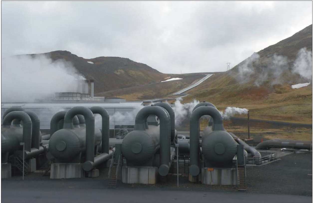
Fig. 8: Hellisheidi, the third-largest geothermal power plant in the world (the southwest Iceland) (Photo: B. Frantál)
