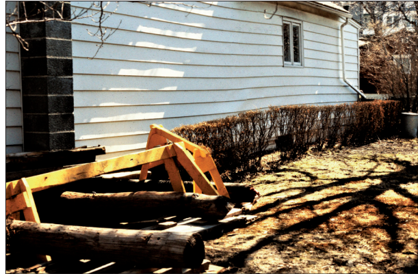
Fig. 2: Abandoned house damaged by subsidence from underground coal mines in Wilkes Barre, Pennsylvania, USA. Photo: M. Pasqualetti
